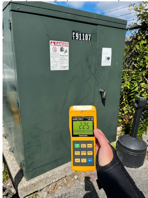
PHOTO #4: Elevated A.C. magnetic field measurements recorded near transformer located on the North side of the property.
